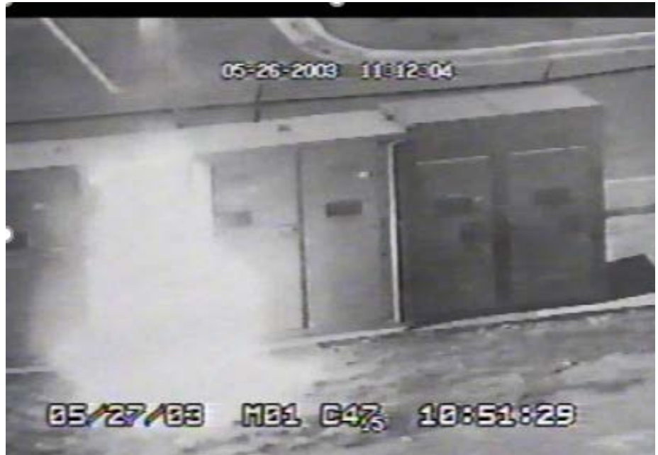
Figure 2: An arc flash hazard is defined as (per NFPA 70E, 2018): A source of possible injury or damage to health associated with the release of energy caused by an electrical arc. Electrical arcs occur whenever there is a short/open, ground fault, or bolted fault across multiple phases.
