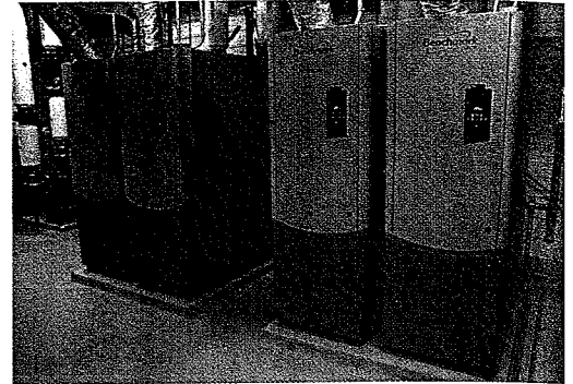
High-efficiency boilers installed at Sweetwater Sound.
