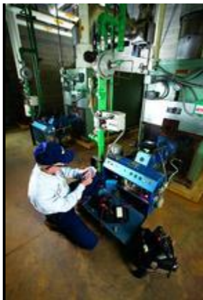
A Linc Mechanical technician works on a similar project to save another organization money through energy efficiency.
