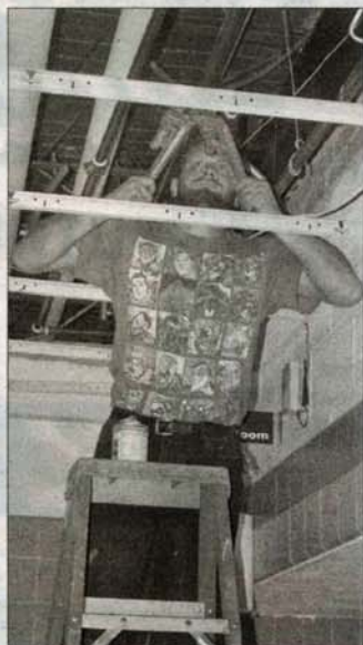
Nick Bell, above, works to install the new piping system as a part of the renovations at Northwest Area High School.
