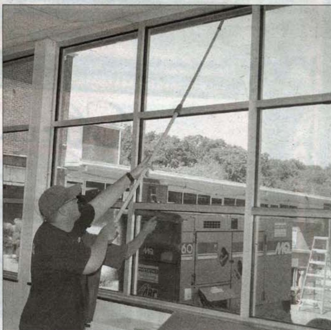
Bill Davis, an employee of PJ's Window Cleaning, is busy cleaning the newly installed windows at Northwest.
