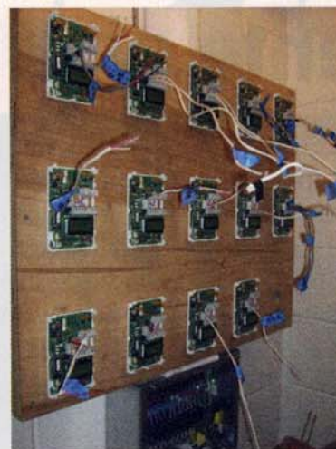
Warehime Hall's control system.
